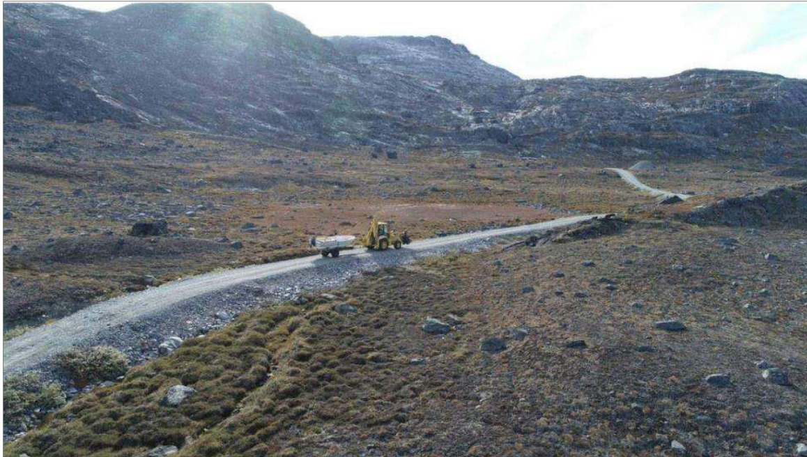
Figure 79: Example of dirt road through terrain (2022 - an access road related to the Buksefjord hydropower facility).
